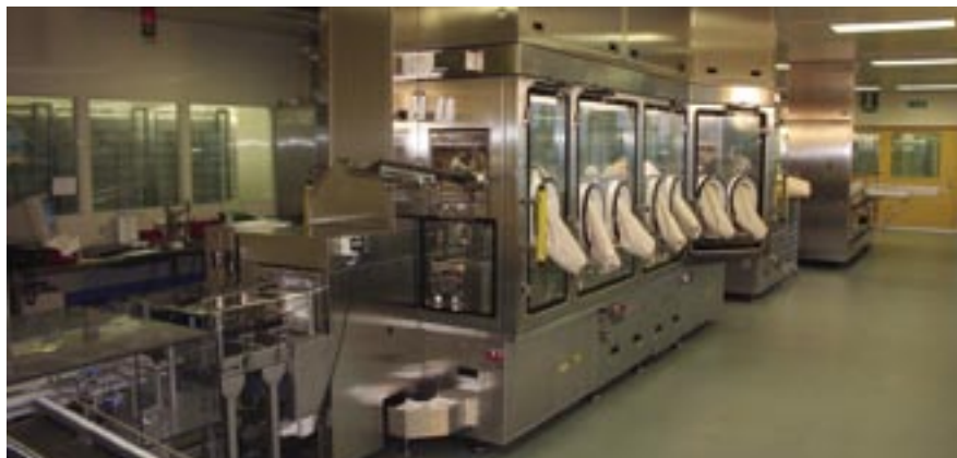
Photo 1: Solvay Pharmaceuticals' isolator filling line in The Netherlands
